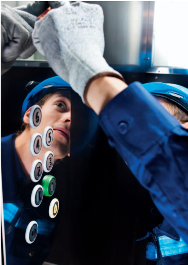
KONE Service Technicians maintain more than one million elevators, escalators and doors worldwide, from both KONE and other manufacturers.
